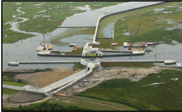
Lake Borgne Barrier, New Orleans. Overall aerial view of radial sector (horizontal rotating) barrier. Source: USACE,
