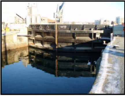
Miter gate in closed position.
