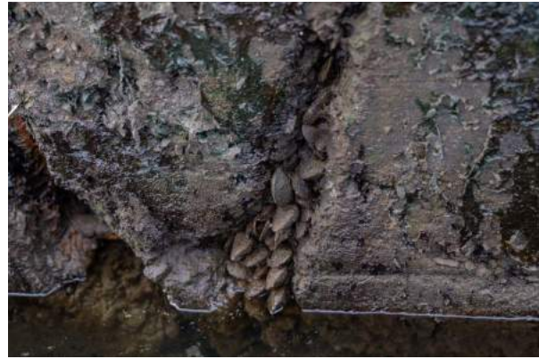
Mussels in concrete southern wall
